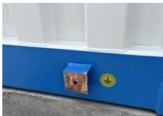
Figure 6 Partial view of grounding copper bar
